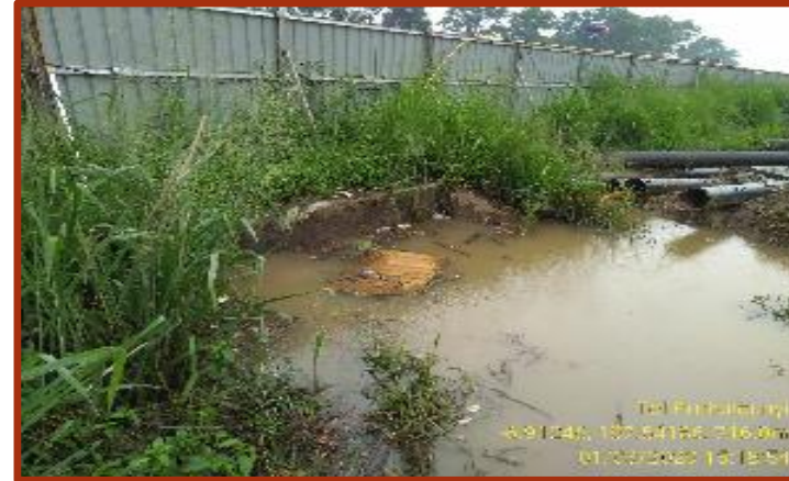
Cross drain tersumbat
